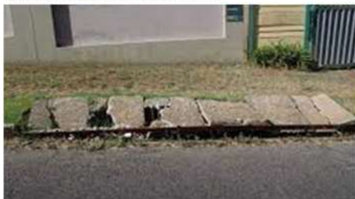
DISLODGED / BROKEN KERB INLET (KI) on Storm water drains
